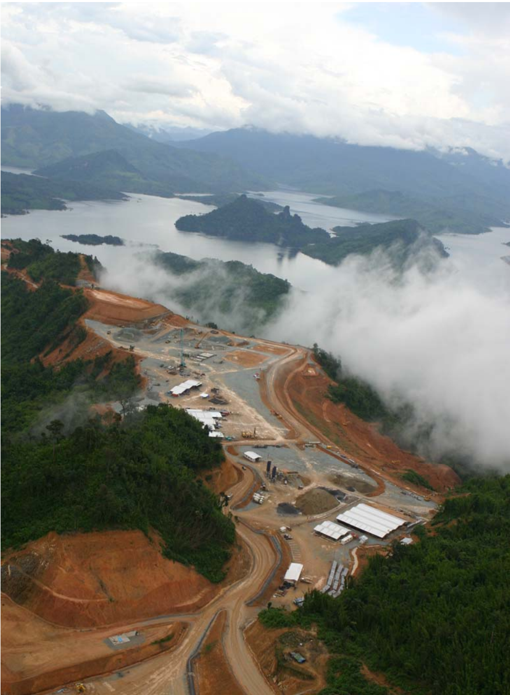
Ban Houayxai plant site with the new Nam Ngum 2 reservoir in the background, October 2010
