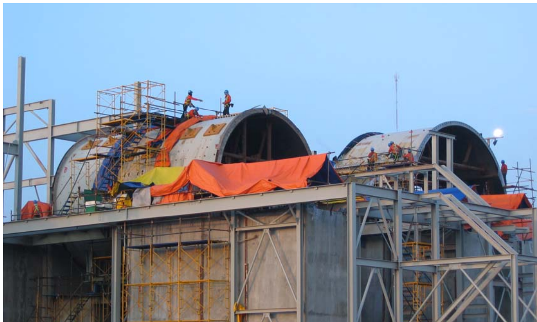
Ball mill (left) and SAG mill (right) in position – photo taken early October
