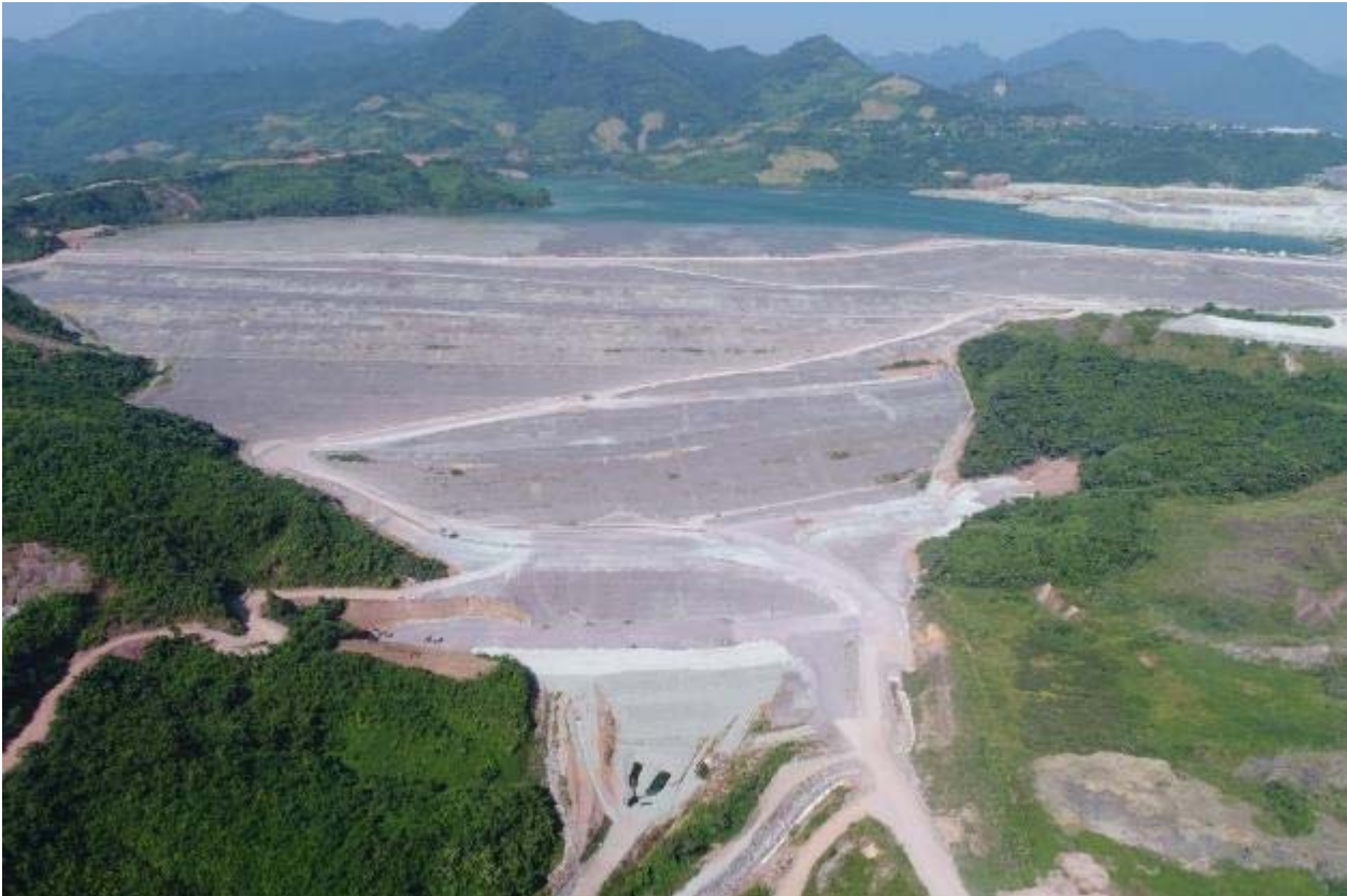
FIGURE 5 - Phu Kham TSF embankment downstream construction with waste rock dump in upper right
