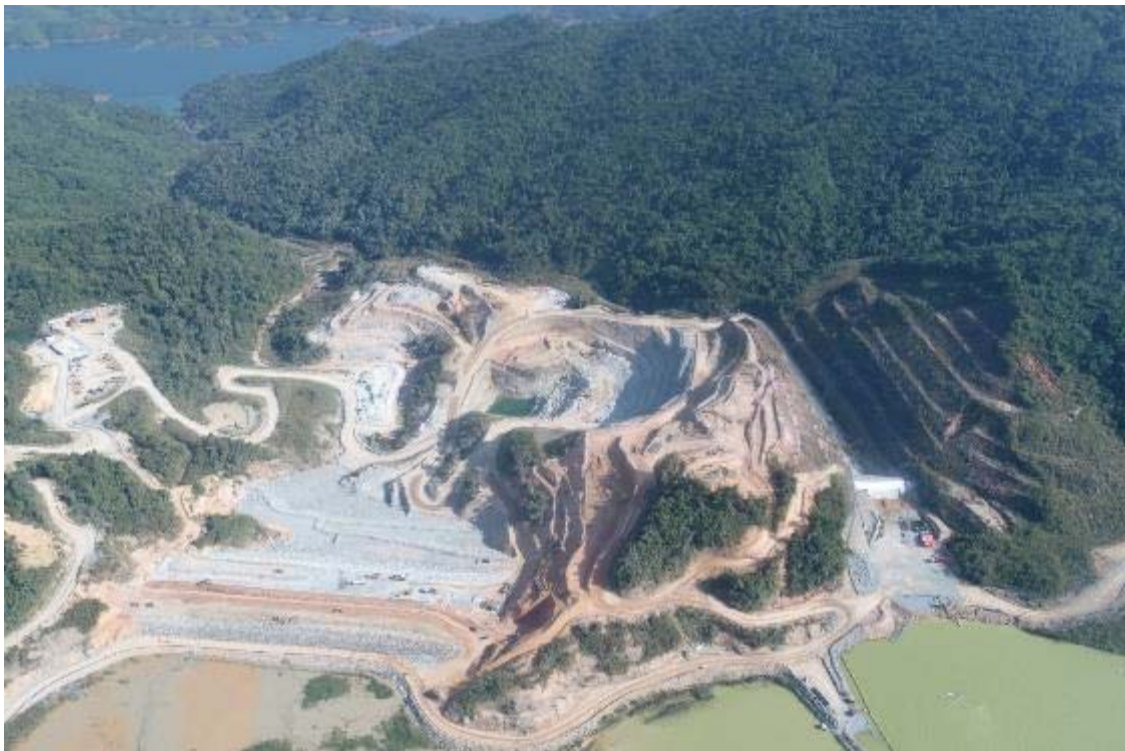
FIGURE 3 - Ban Houayxai TSF embankment, construction quarry and spillway with tailings in foreground
